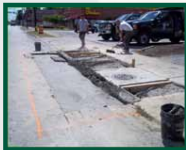
On SOM Center Road our crews installed catch basins, curb & road restoration.
